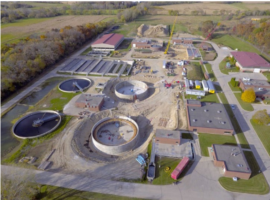
Figure 6.3. The Sun Prairie Wastewater Treatment Plant under additional construction (Photo credit: City of Sun Prairie, October 2020)
